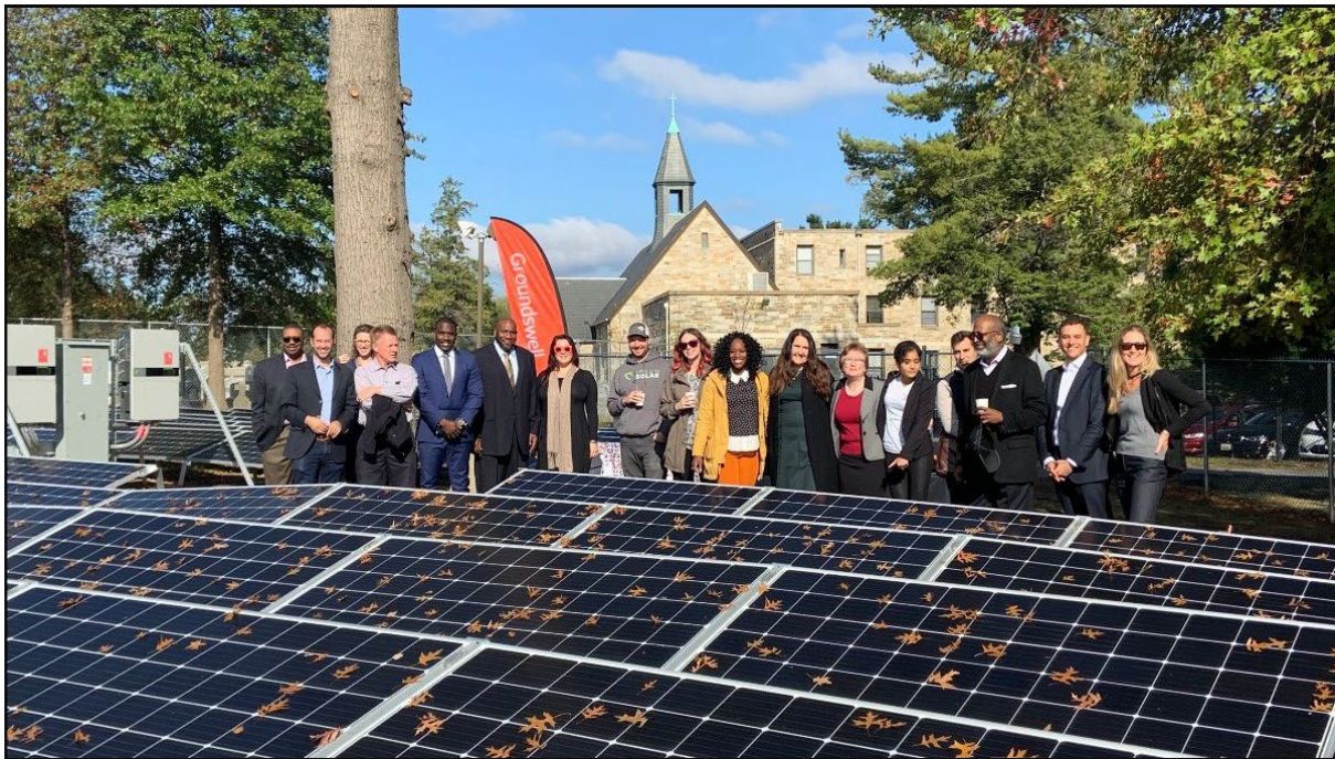
NYCEEC-SunLight General Capital solar project for a Washington, DC house of worship. Photo credit: SunLight General Capital
